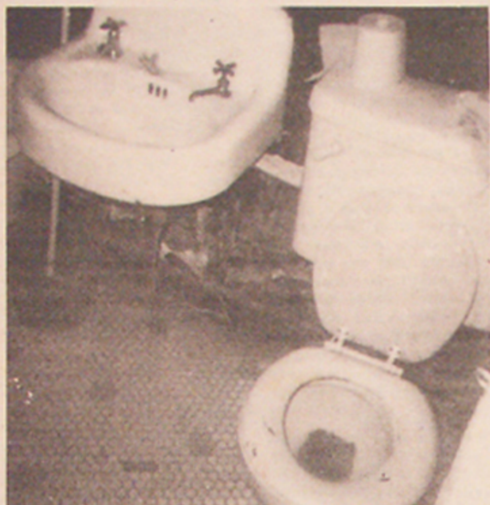
One of many bathrooms with rat holes under sinks. (Rats paradise).
